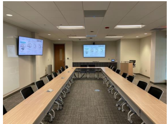
For each of the five conference rooms, UWCA installed an integrated ClearOne AV solution using the CONVERGE Pro 2 with the patented BMA CT and high-definition UNITE pan-tilt-zoom cameras.
